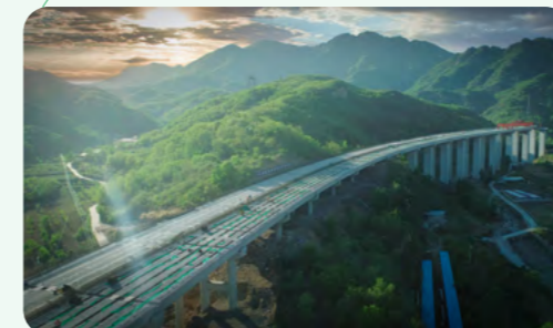
首都地区环线高速公路承德（李家营）至平谷（冀京界）段项目 Project from Chengde (Lijiaying) to Pinggu (Beijing-Hebei boundary) of Ring Expressway in Capital Region
